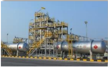
Hydrogenation Plant (Brunei)
